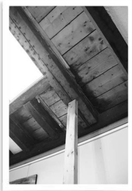
Roof repairs needed
